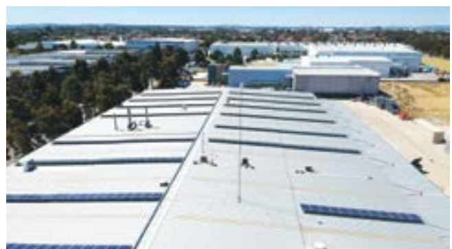
Solar panels installed at McConnell Seats Australia Pty Ltd's plant
