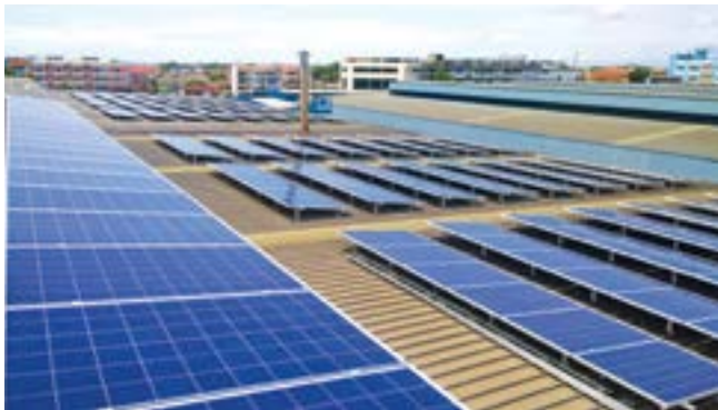
Solar Panels installed at APM Springs' plant
