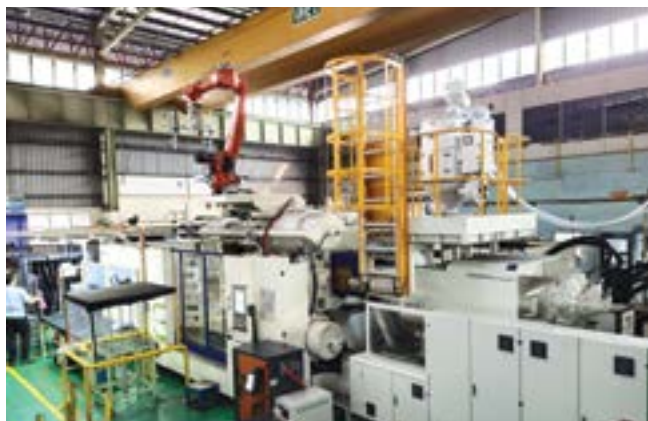
New Injection Machine installed at Bukit Beruntung plant
