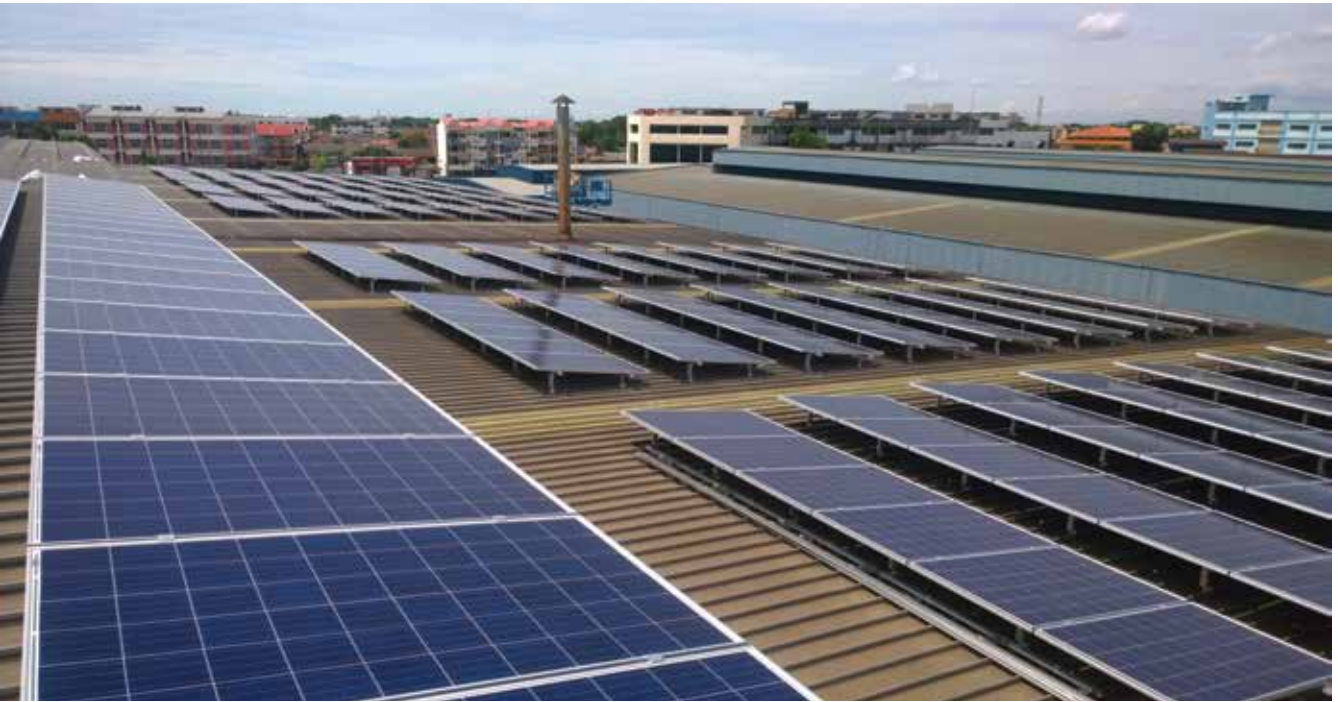
Solar Panels installed at APM Springs' plant
