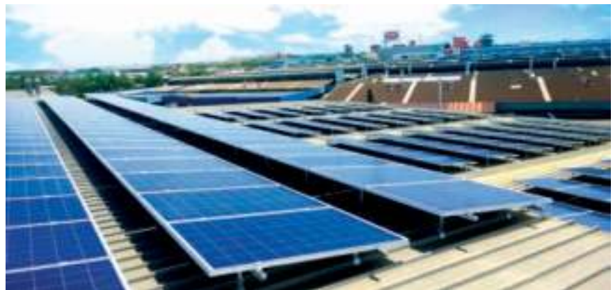
Solar Panels installed at APM Springs' plant
