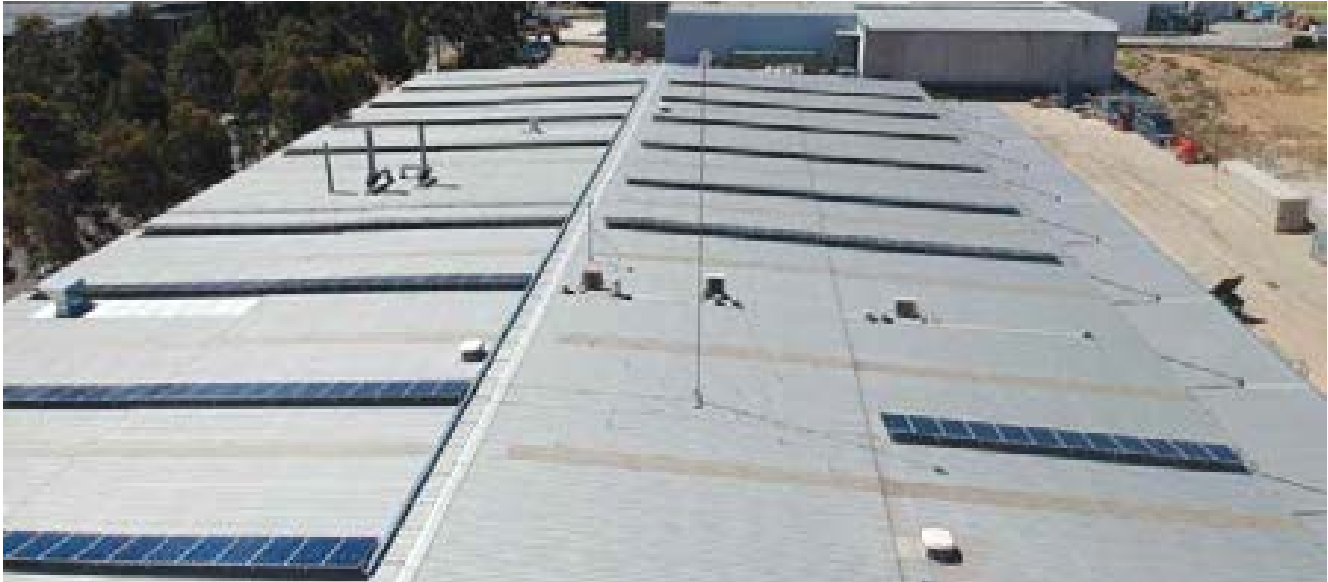
Solar panels installed at McConnell Seats Australia Pty Ltd's plant
