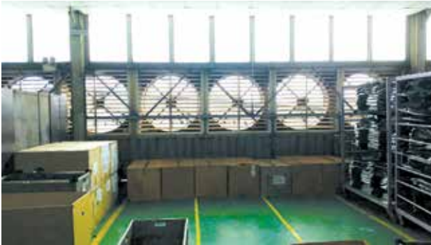
Evaporative Cooling System
